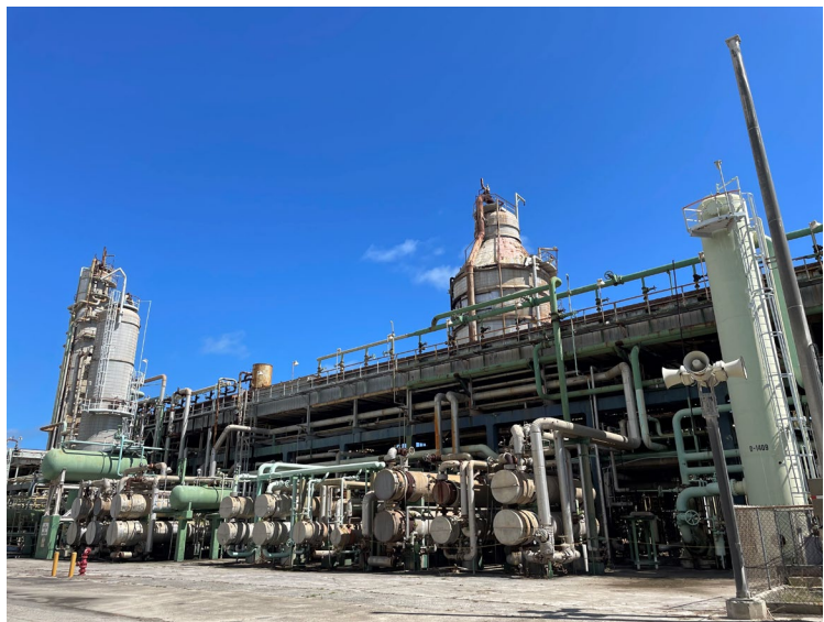
No. 3 Crude Distillation Unit and No. 1 Vacuum Unit
