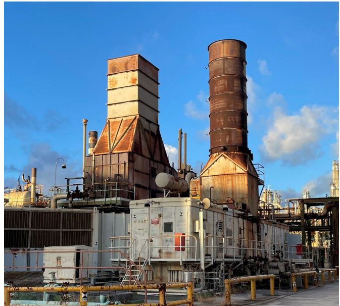
No. 4 Gas Turbine
