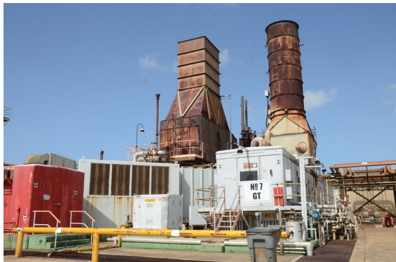
No. 7 Gas Turbine
