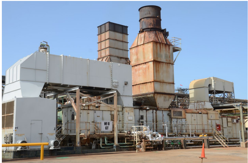
No. 8 Gas Turbine
